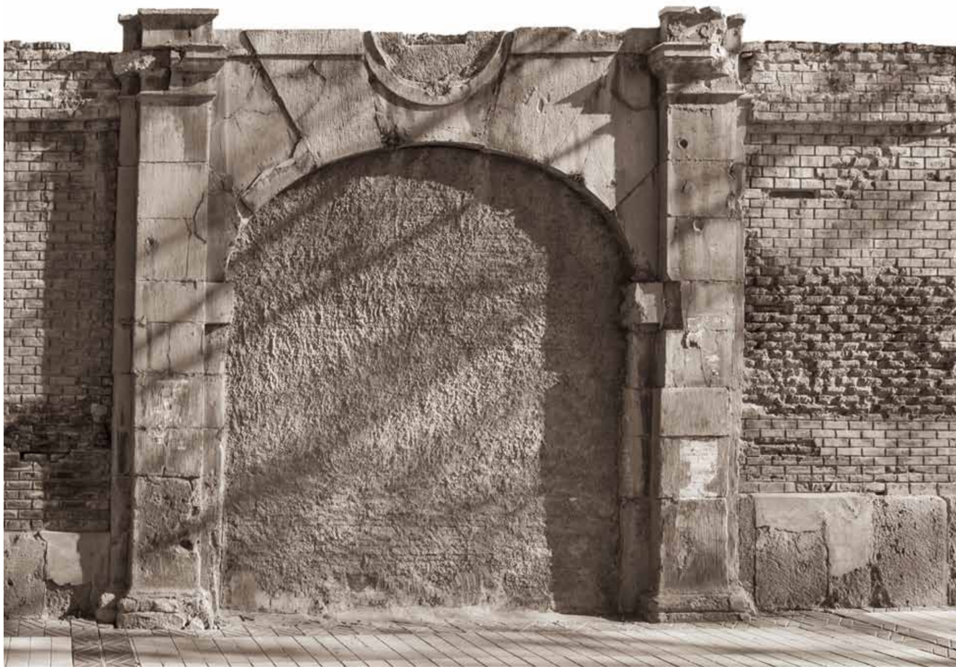
Canvas of the former Cavalry barracks, called "Cuartel del Cid", in front of the Averly factory. Present state.
